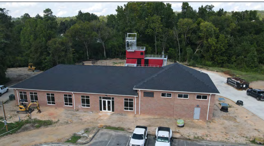
Phenix City's new fire training facility features a training classroom, offices and an apparatus bay. The new fire drill tower in Phenix City offers firefighters critical hands-on training. Photo credits: Phenix City Economic Development Department
